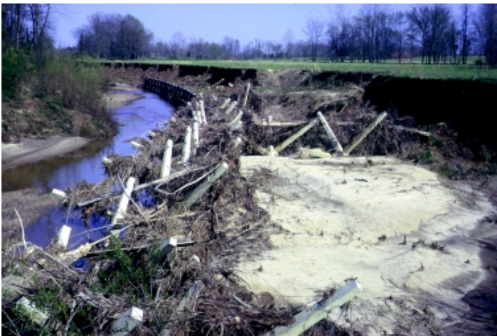
Figure 16-31 Concrete jack system several years after installation
